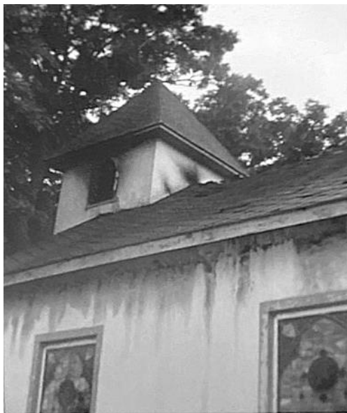
Some of the exterior fire, smoke, and water damage to the Chapel
