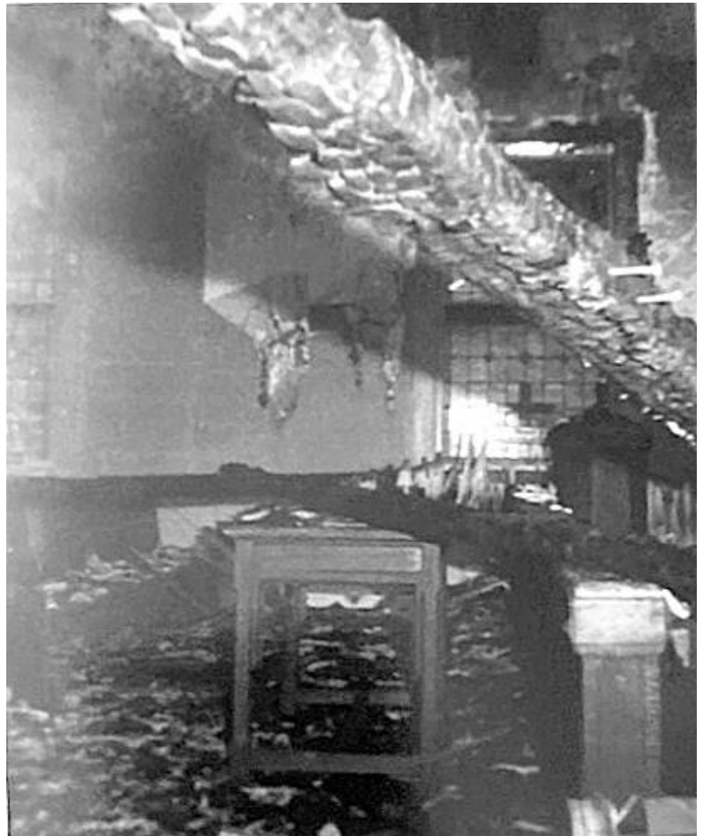
The extensive interior damage to the Chapel
